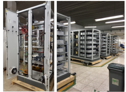
Fig. 4. TF power supply charger (left) and part of the TF ultracapacitor banks (right).
