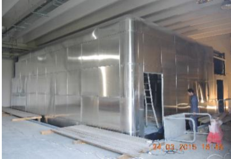
Figure 4.123: High voltage deck hosting all the power supplies and diagnostics dedicated to the plasma source
