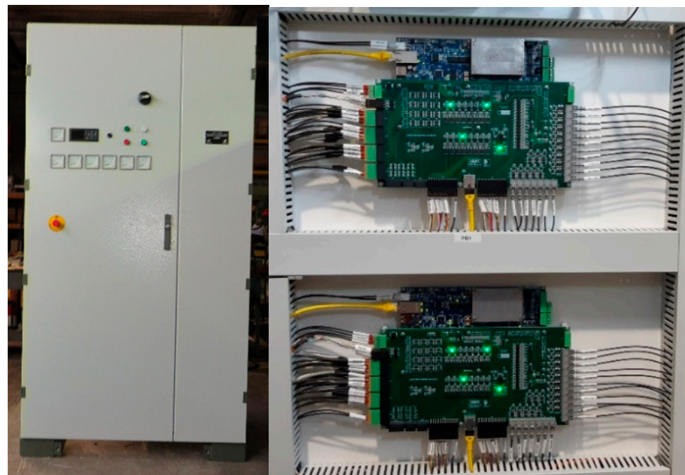
Figure 5. Charging station with integrated power electronics converters and control platforms.
