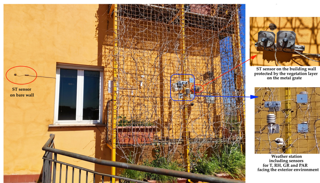
Figure 2. Section of the building at ENEA Casaccia RC showing the steel infrastructure sustaining vegetation in the SW façade at the first-floor level. The picture was taken in March, when the deciduous Parthenocissus quinquefolia (L.) Planch. Was still bare after losing its leaves in winter. On the
