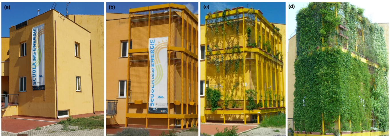
Figure 1. Consecutive steps in the installation of the green wall at the ENEA “green” building demonstration platform. (a) The building without the vertical green wall installation; (b) yellow stainless-steel infrastructure with three series of planter holders, respectively at the base and on the 1st and 2nd floor of the building; (c) transplanted plants attaching themselves to the lattice infrastructure (April 2017); (d) plants completely covering the infrastructure (June 2019).
