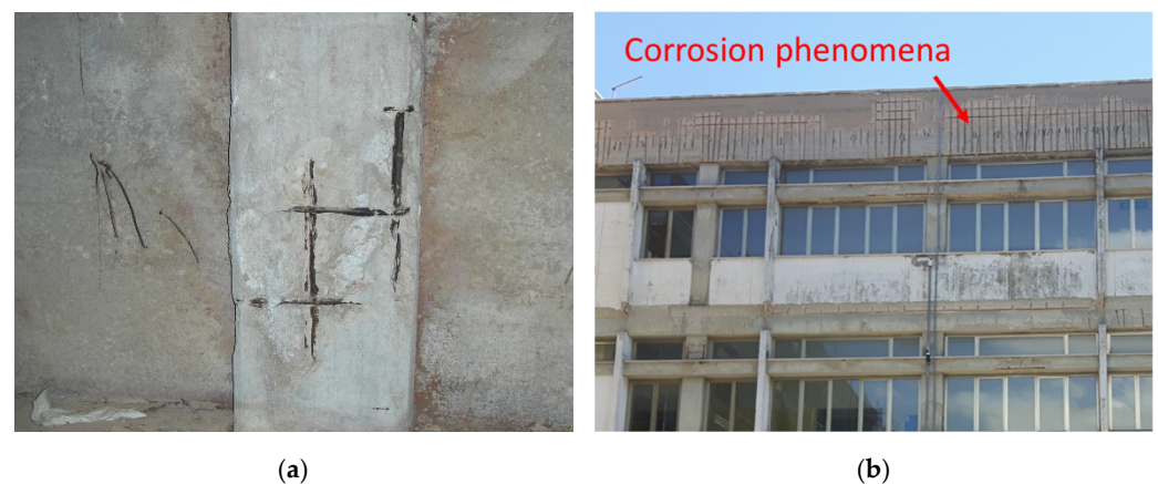
Figure 6. Example of corrosion phenomena to a column in the basement (a) and façade structural members (b) observed during in situ surveys (from UEFA/ELENA research project [23]).
