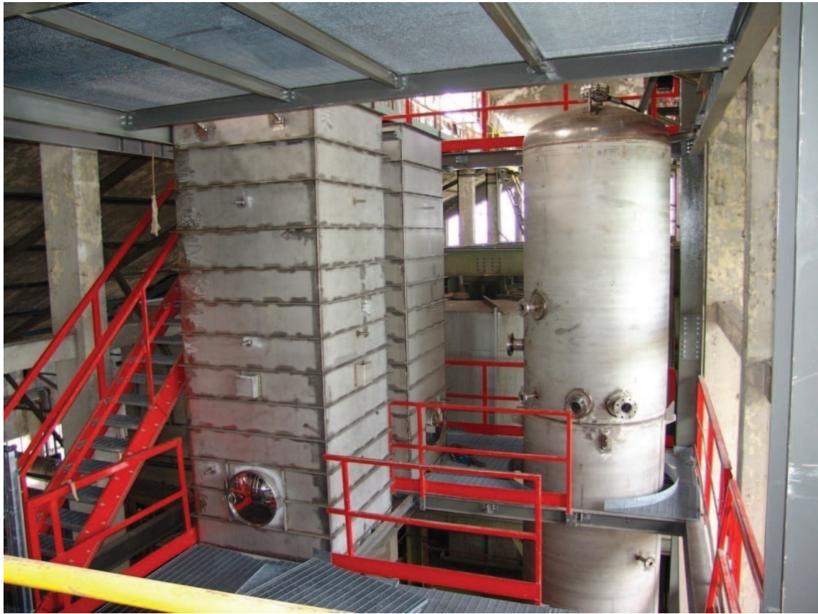
Figure 4 – SPES 3 condenser pool: side view
