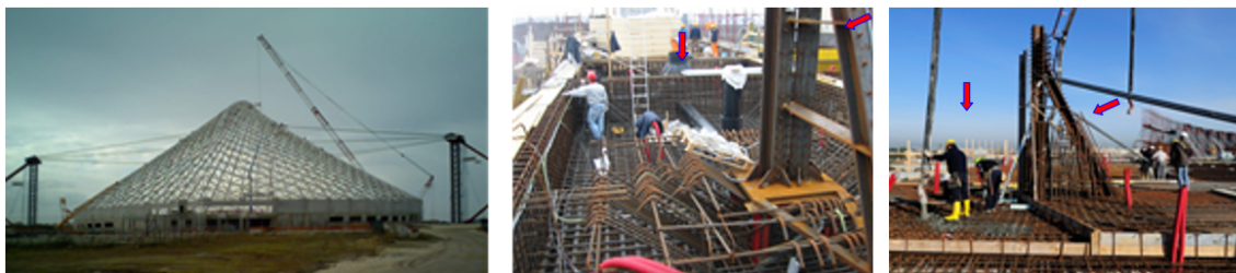
Figure 1. The sports complex during the construction works with the fan-shaped roof without glass tiles in position (left). Construction works at the location of the mezzanine and pillar (centre and right). Arrows provide reference to locate the components in figure 2.
