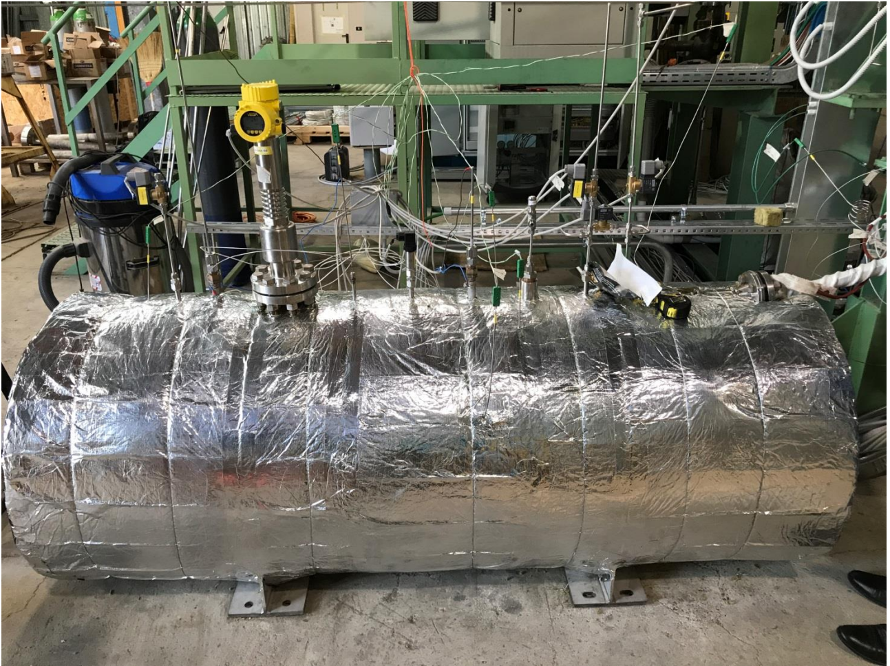
Fig. 2—5 – S4_A storage tank.
