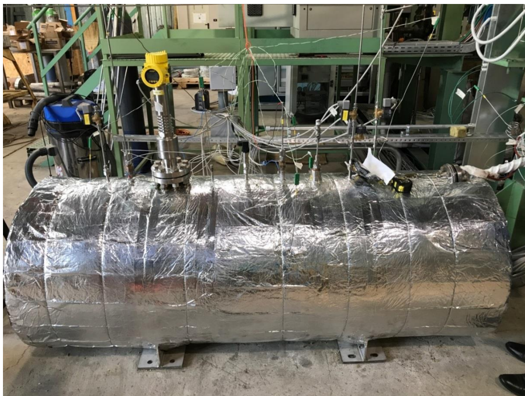
Fig. 8 – S4A storage tank.
