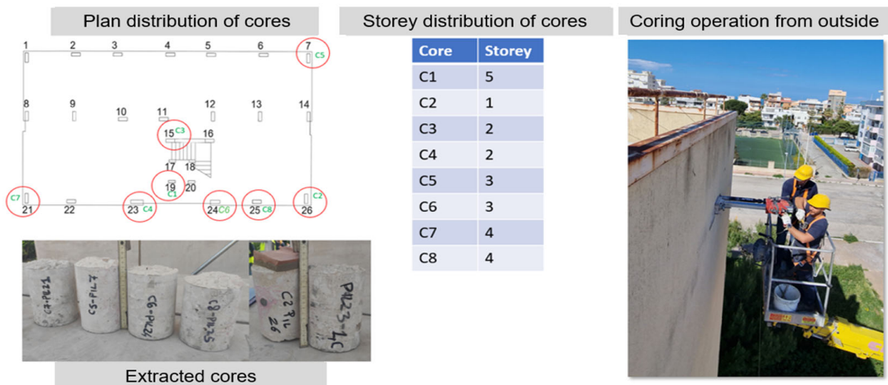
Figure 10. Concrete core drilling (for column and storey numbers, see Figures 2 and 3 respectively).
