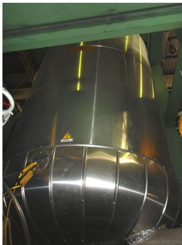
Fig. 9 – S3V dump tank.
