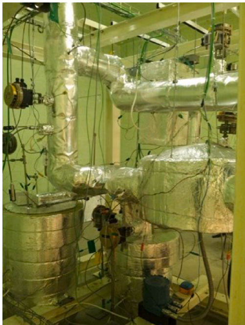
Fig. 2. Overall view of Lifus 6 plant.
