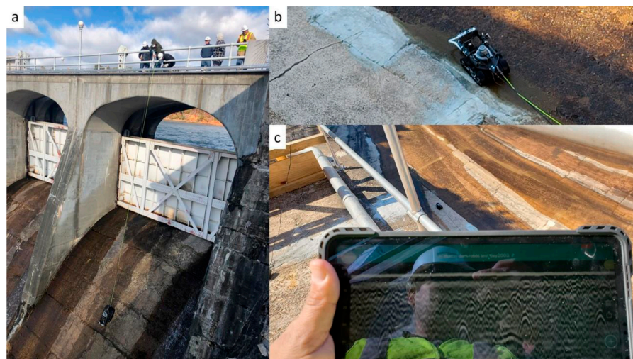
Figure 9. (a) Crawler with GPR being lowered onto spillway; (b) Crawler with GPR collecting data across repaired concrete surface; (c) Data collection with handheld device [82].
