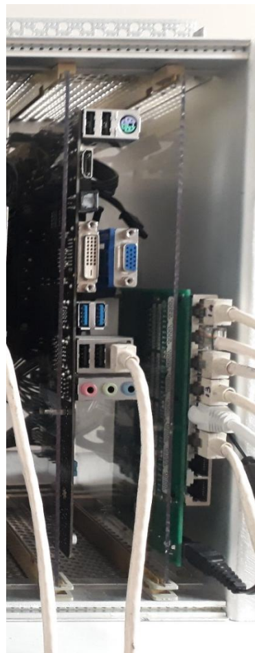
Fig. 11: Network switch mounting.
