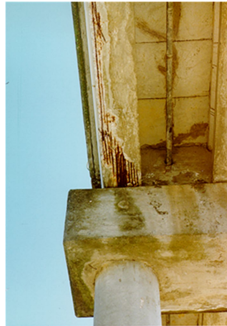
Fig. 5 Reinforcing bar exposed in proximity of the support
