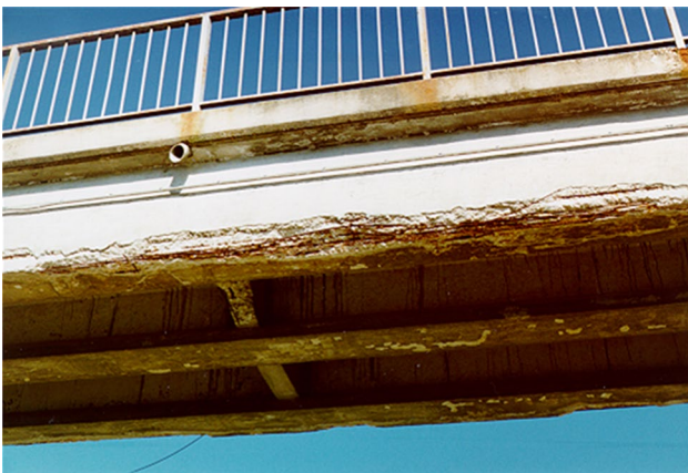
Fig. 4 The carbonation of the concrete and the reinforcing bar exposed
