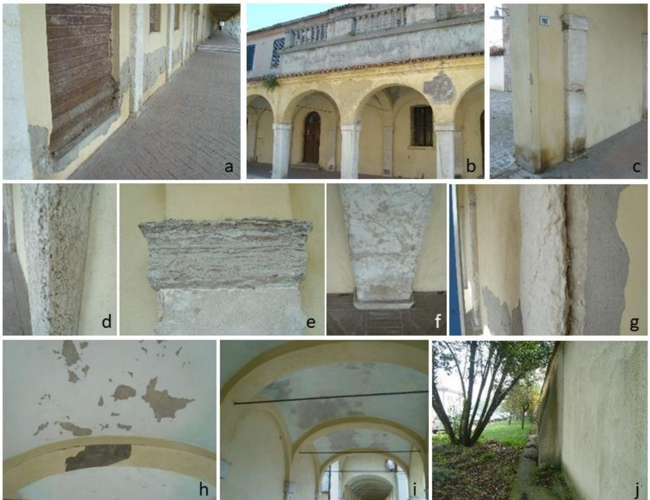
Figure 3. Degradation phenomena observed on the Loggiato dei Cappuccini during the analysis campaign on summer/autumn 2015: (a) degradation of the plaster placed on the internal wall; (b) lack of material on the external wall; (c) black crust at the base of the column; (d) alveolization phenomenon on the columns; (e) physical disintegration on the top of the columns; (f) physical disintegration on the basement of the columns; (g) flaking of the columns along the sedimentation floors; (h,i) degradation of the painting layer; (j) degradation caused by trees.
