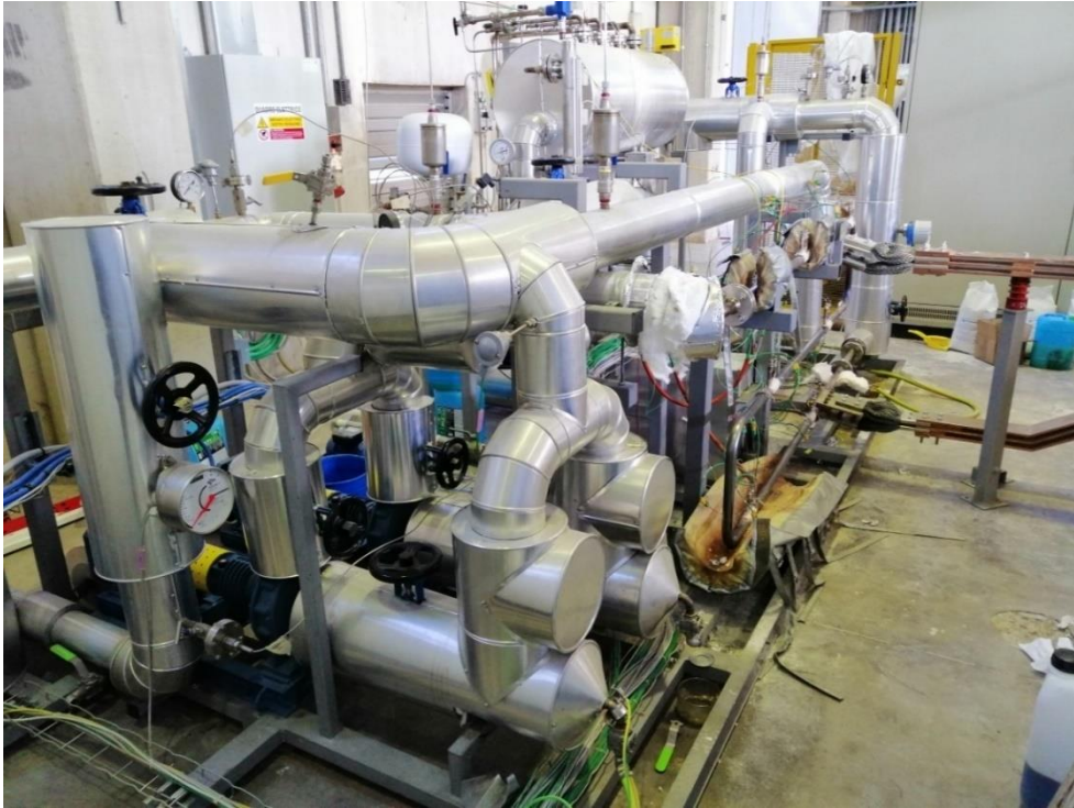
Figure 7. Experimental plant: overall view.
