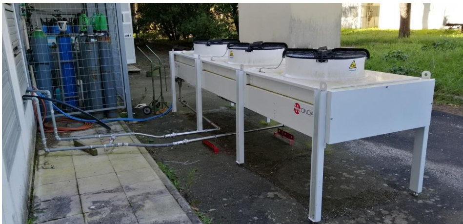
Figure 2. Experimental plant: Air Cooler system.
