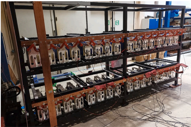
Fig. 12. Varistor frame during the test at higher current in KEMA laboratory.
