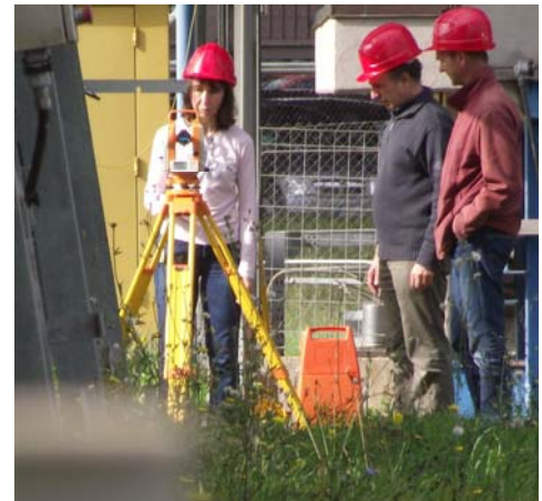
ENEA electronic solar compass used during the alignment of a solar concentrator.
