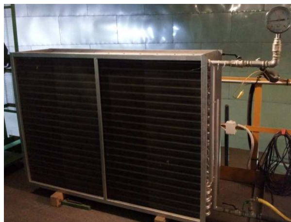
Figure 3.3: Fan cooler of the secondary circuit
