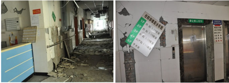
Fig. 14.10 Damage suffered by the two conventionally founded buildings of the hospital of Fig. 14.9 (Zhou et al. 2013)
