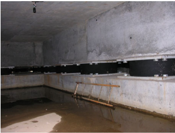
Fig. 14.13 Some of the 193 HDRBs, manufactured in Italy, which protect the building of Fig. 14.12 (picture taken on September 23, 2011, during the 2011 Sochi Conference) (Martelli et al. 2012a)
