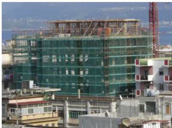
Fig. 14.19 Eight-storey isolated building which is nearing completion in Messina on 22 LDRs and 2 SDs. Its structural safety will be certified by A. Martelli in 2014
