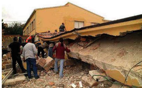
Fig. 14.14 Francesco Jovine school of San Giuliano di Puglia, after its collapse during the 2002 Molise & Puglia earthquake ( M = 5.9 )
