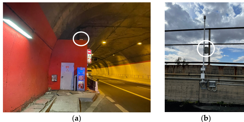
Figure 3. (a) The emergency area of the Galleria San Demetrio where the MONICA IoT sensor node has been installed (in the white circle); (b) the MONICA installed in an emergency area on the viaduct (in the white circle).
