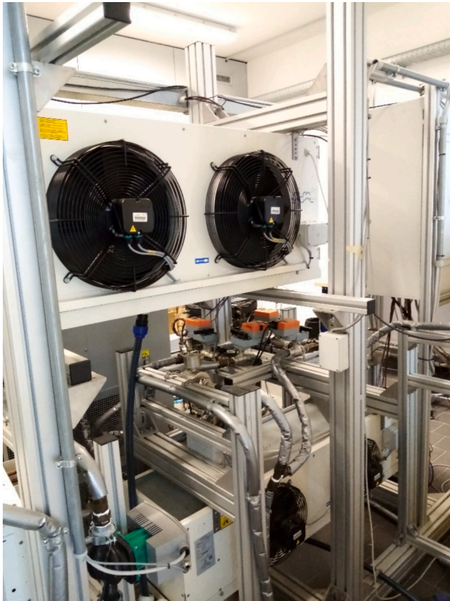
Fig. 3. Heat exchangers used to simulate refrigeration loads.
